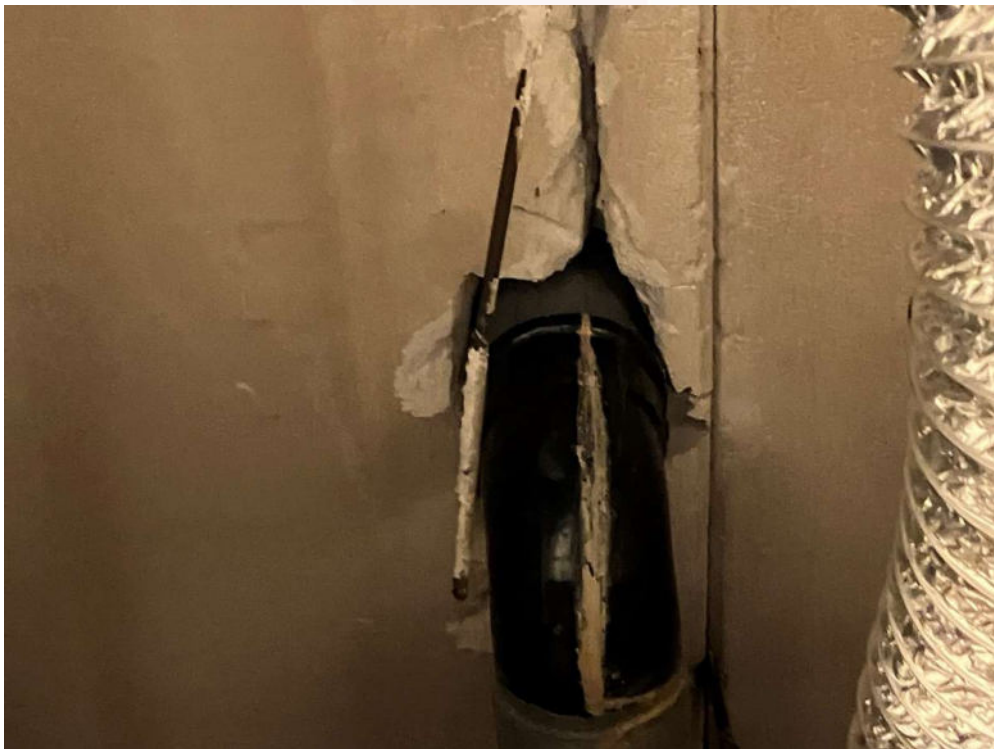
Photograph 38 – Service penetration in RAAC Concrete with no trimming support and bent reinforcement visible – no change
