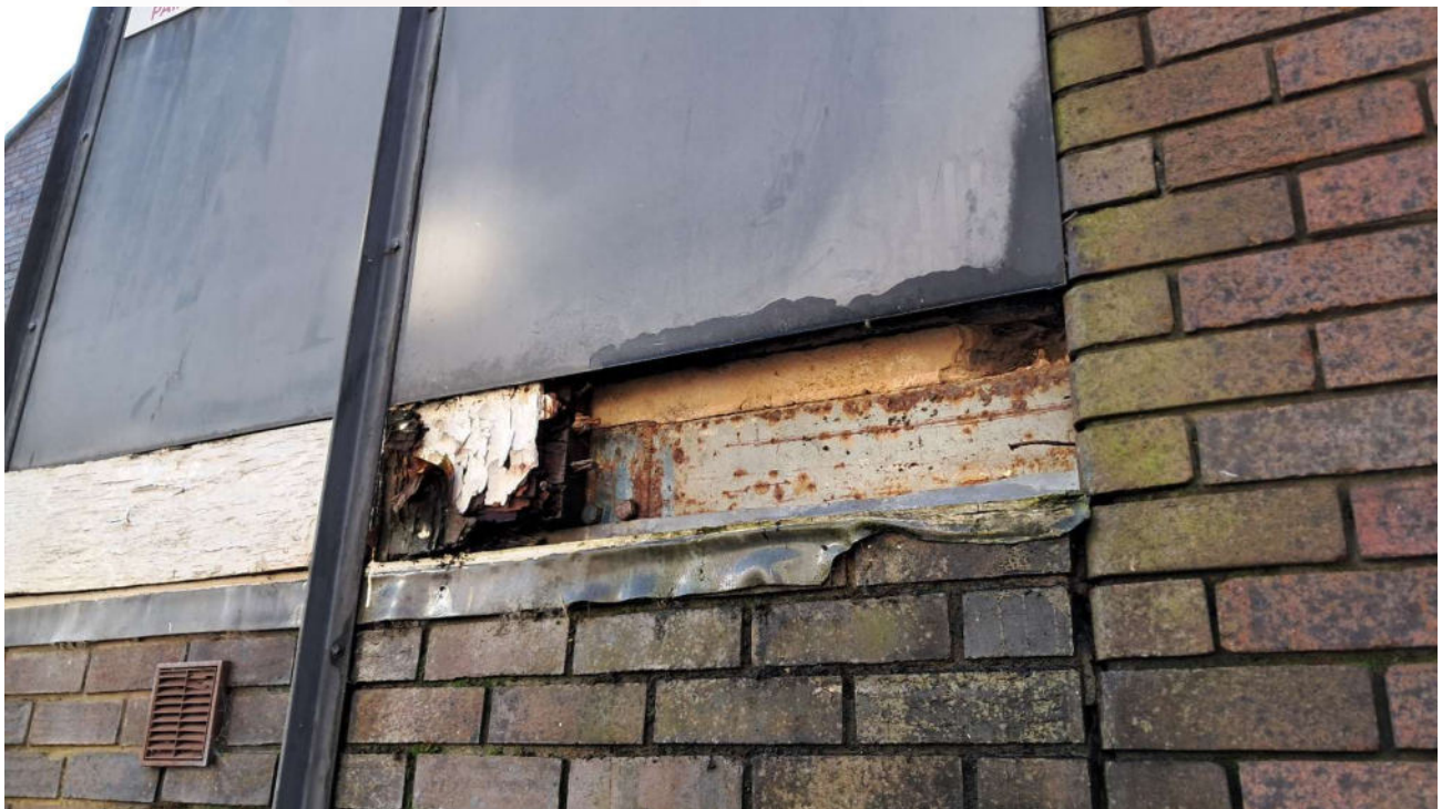
Photograph 11 – Rear elevation of Market Hall close up damage of fascia board
