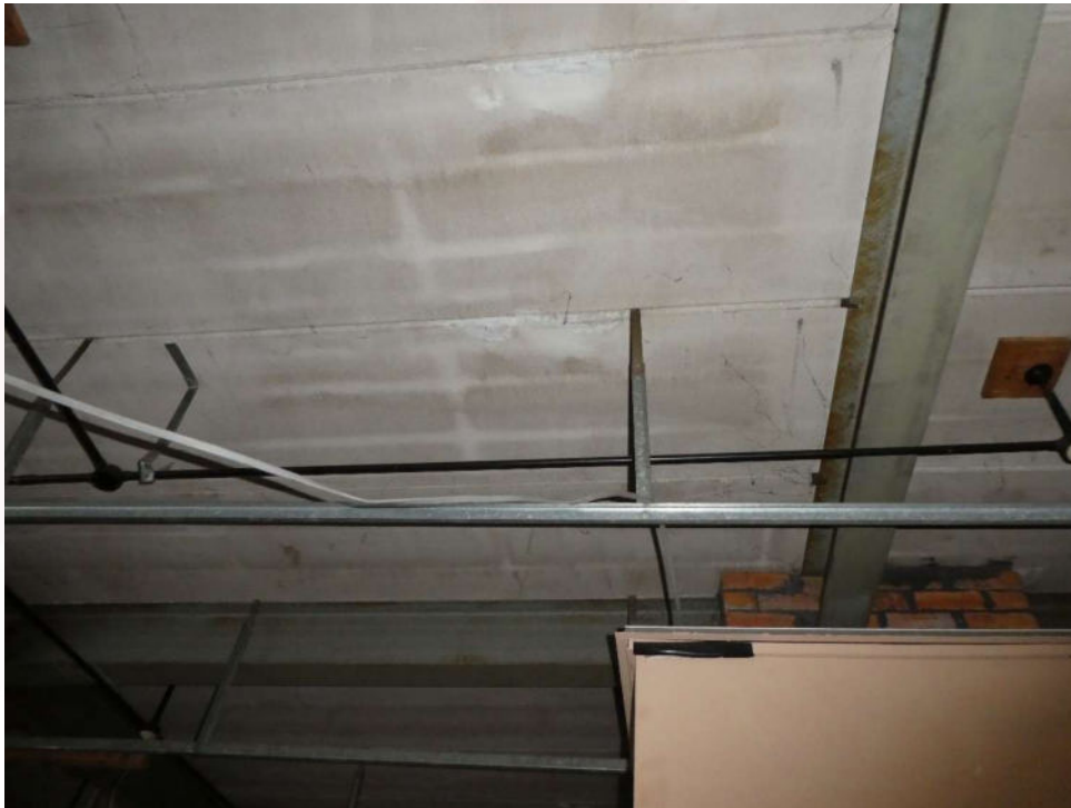
Photograph 35 – Typical condition of RAAC Concrete over Lounge Bar – staining visible
