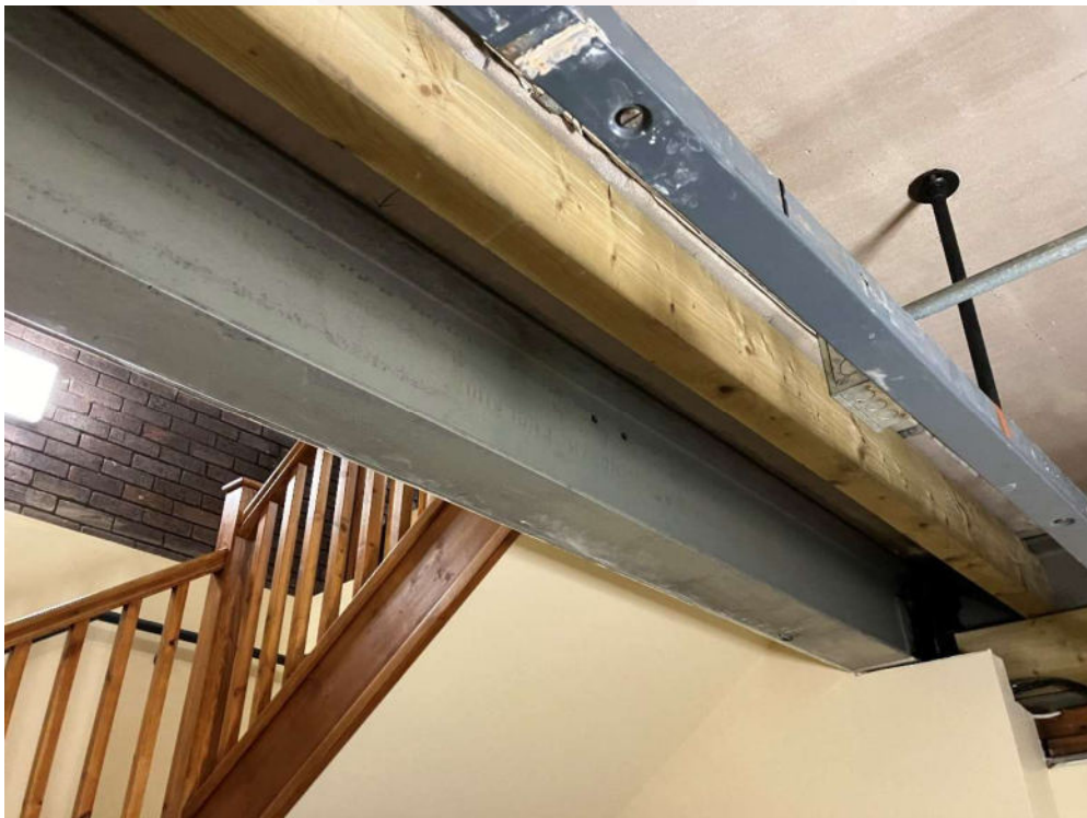
Photograph 48 – RAAC concrete forming landing to fire escape leading from Lounge Bar to Corridor
