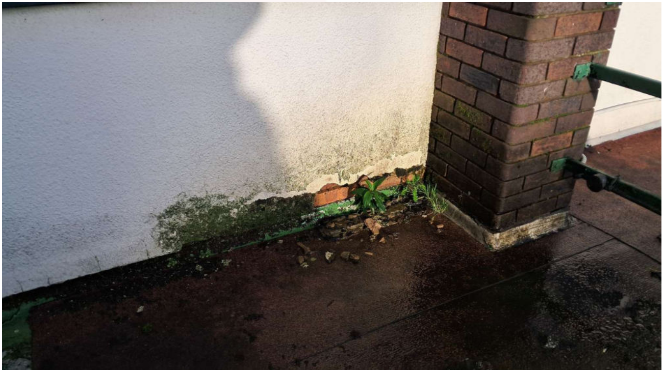
Photograph 17 – Loss of mortar and algae staining
