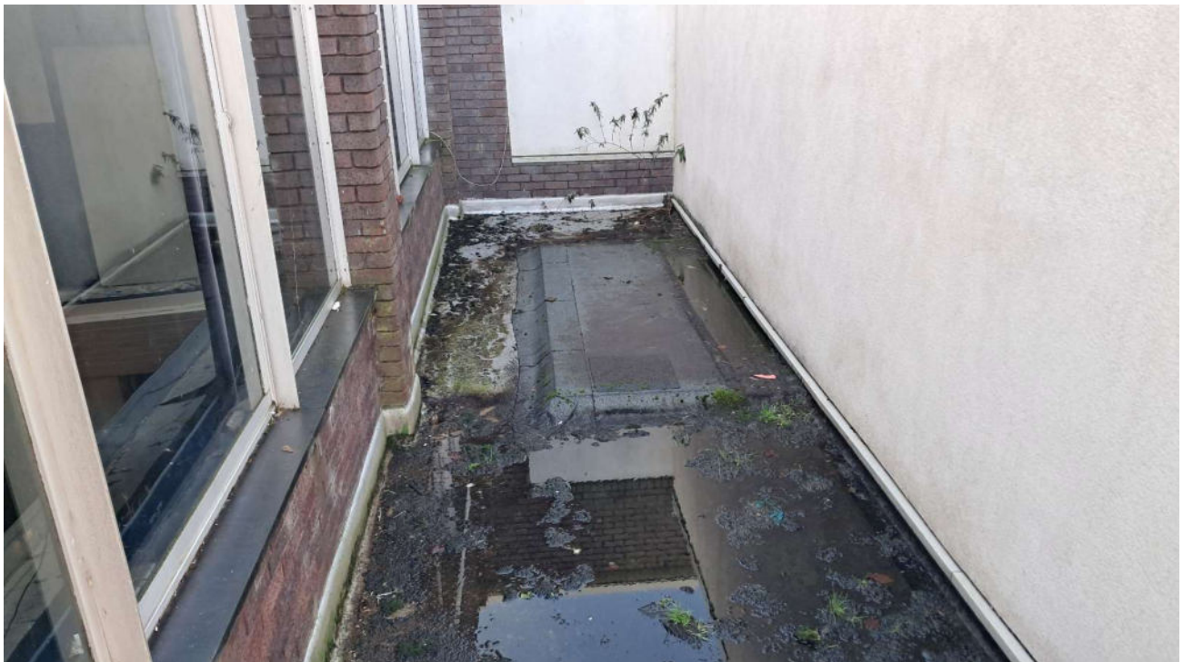
Photograph 19 - Contained roof over corridor with no apparent drainage – standing water
