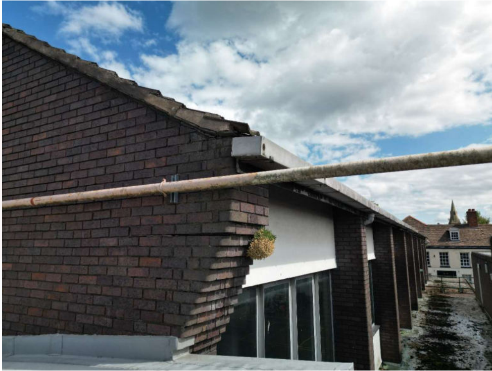
Photograph 18 – Displacement and cracking to corbel on front gable elevation – no change
