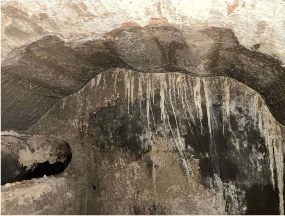
Photograph 33 – Damp to front of basement – no change
