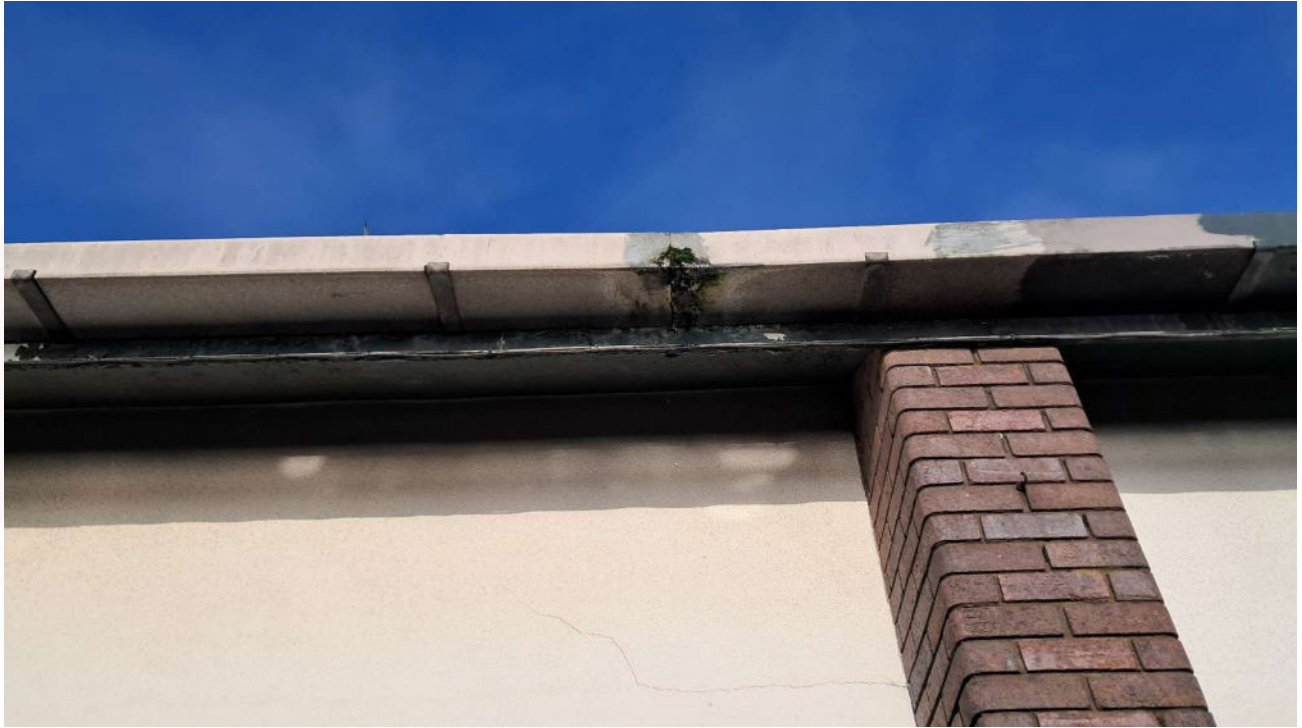
Photograph 16 – Typical cracking to panelling above glazing, leaking gutters
