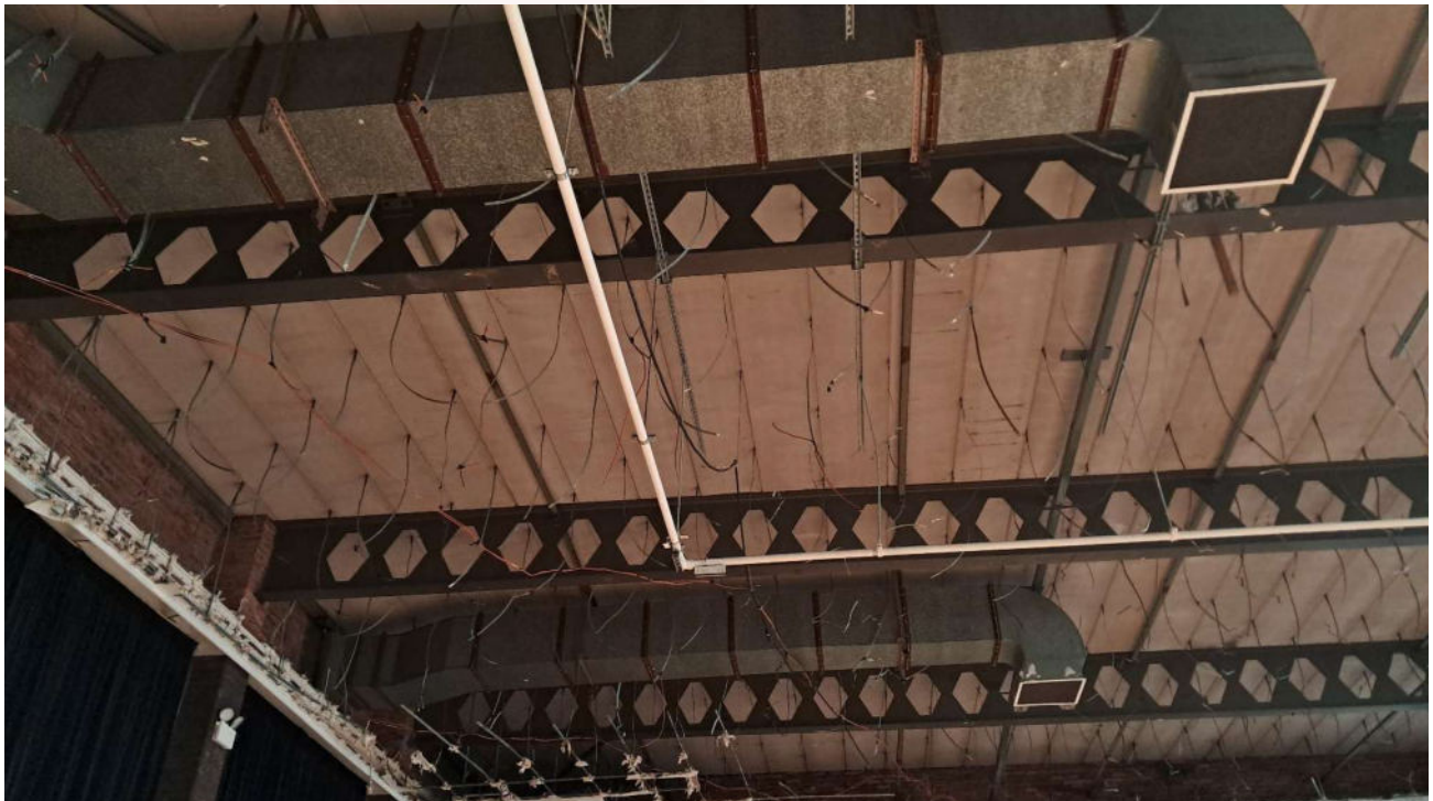
Photograph 40 – roof arrangement over theatre hall – black lateral staining visible to isolated panels
