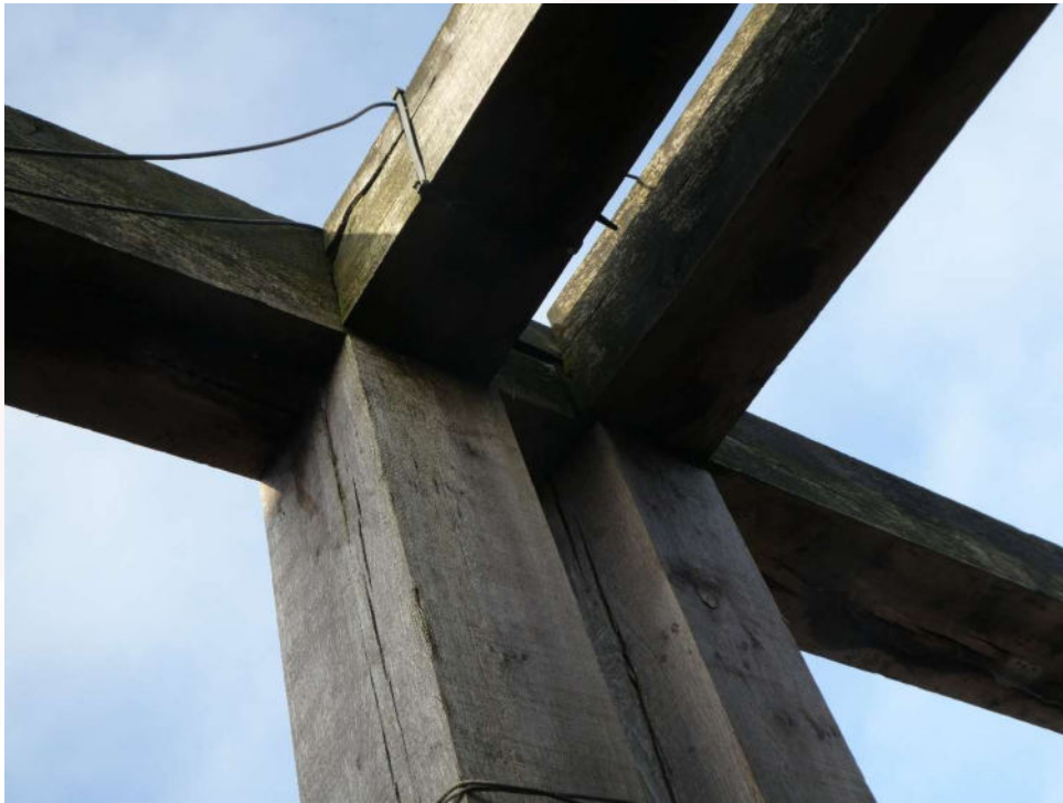
Photograph 51 – splits and twisting to timbers on front balcony
