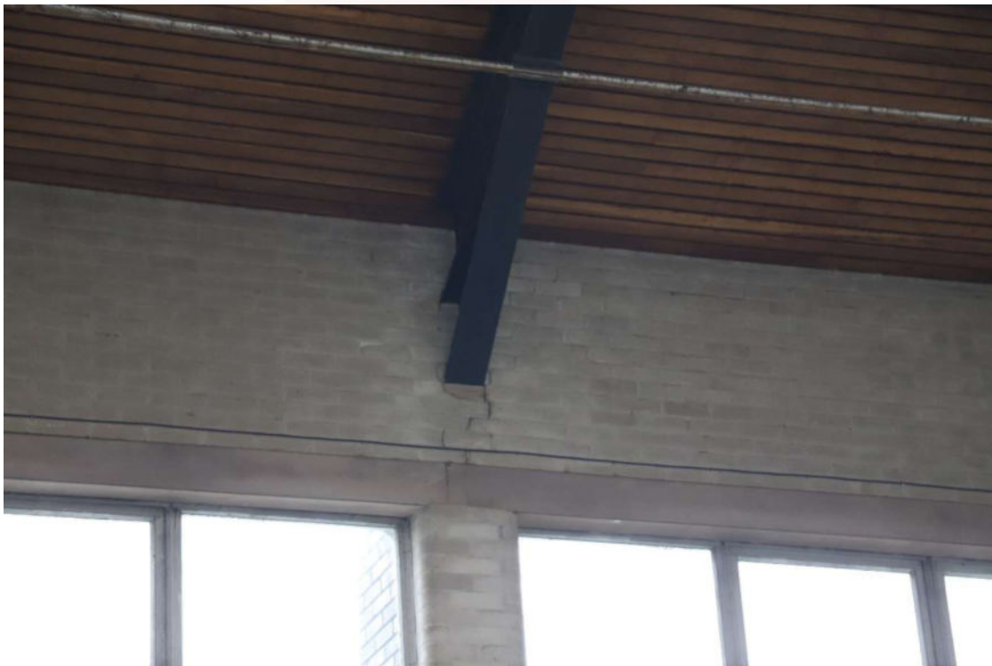
Photograph 42 – Cracking at eaves of Market Hall portal frame – no change
