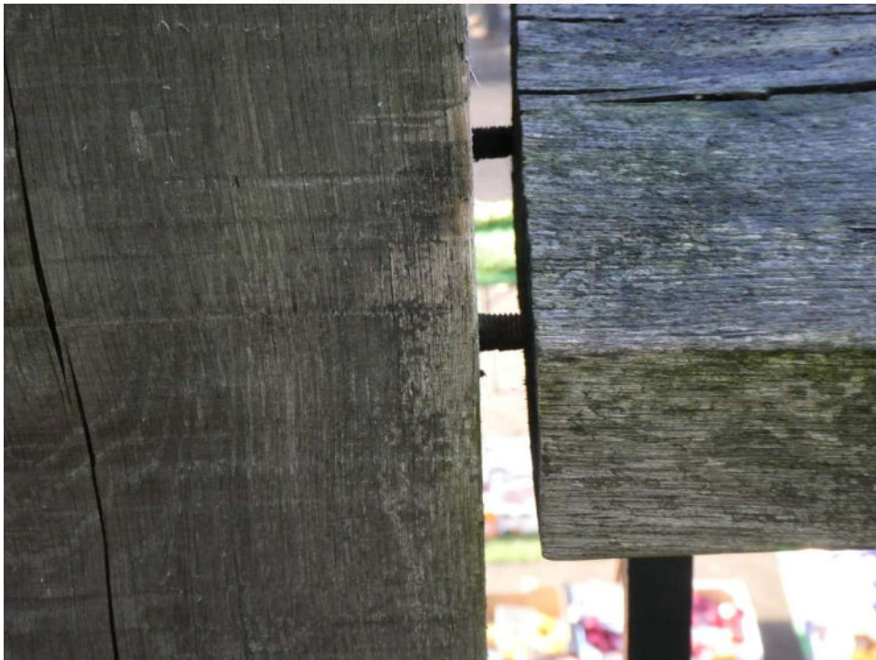
Photograph 52 – separation at balustrade joints
