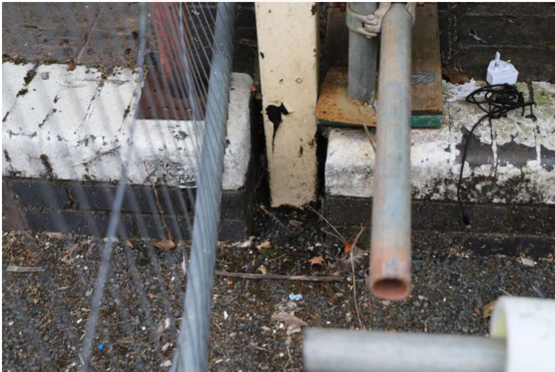
Photograph 7 – Loss of section to base of column supporting canopy in contact with ground – no change
