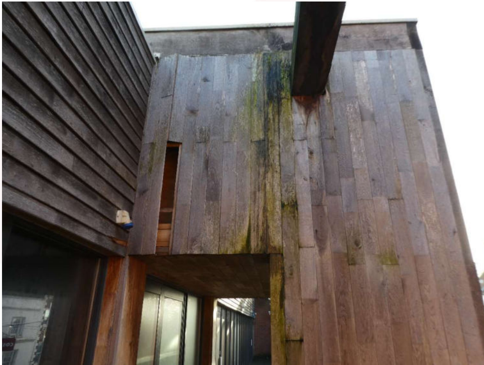
Photograph 53 – staining to cladding and missing panel
