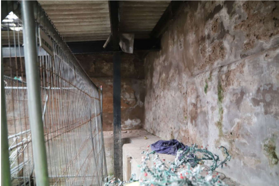
Photograph 49 – Typical damp to rear party wall in stores – no change
