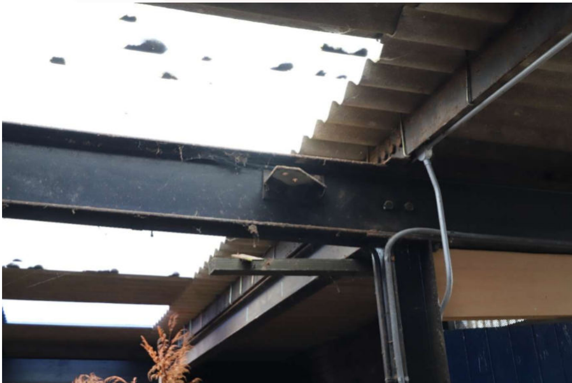
Photograph 50 – Missing bracing to stores – no change
