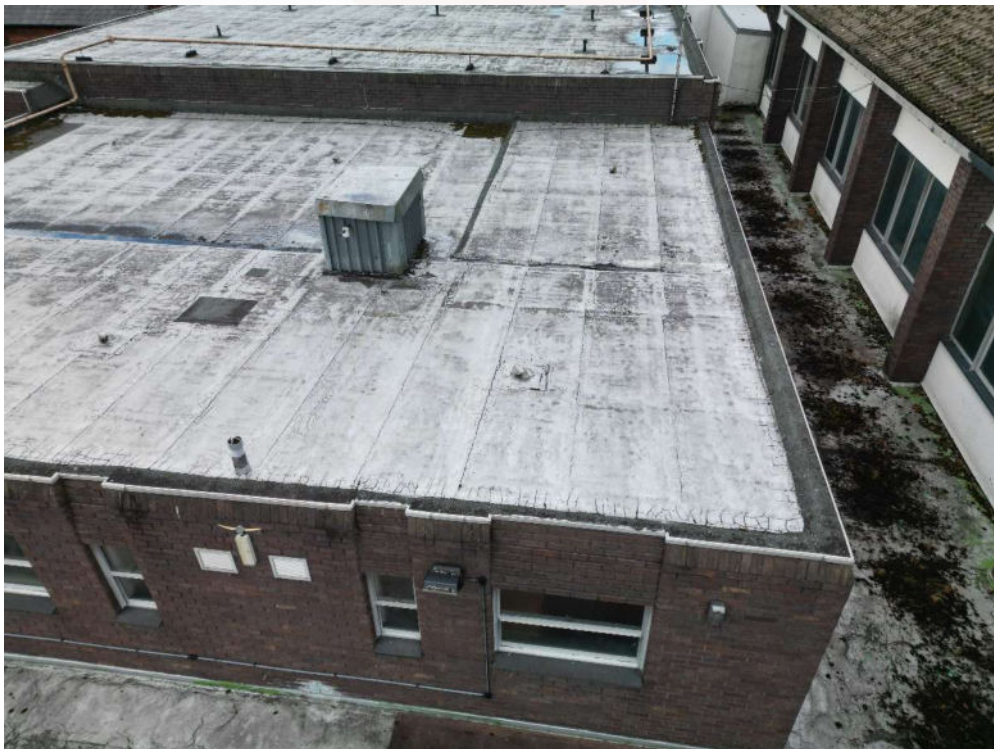
Photograph 25 – Roof over dressing rooms 2024 for comparison
