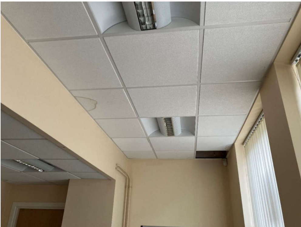
Photograph 34 – evidence of water ingress to offices – no change
