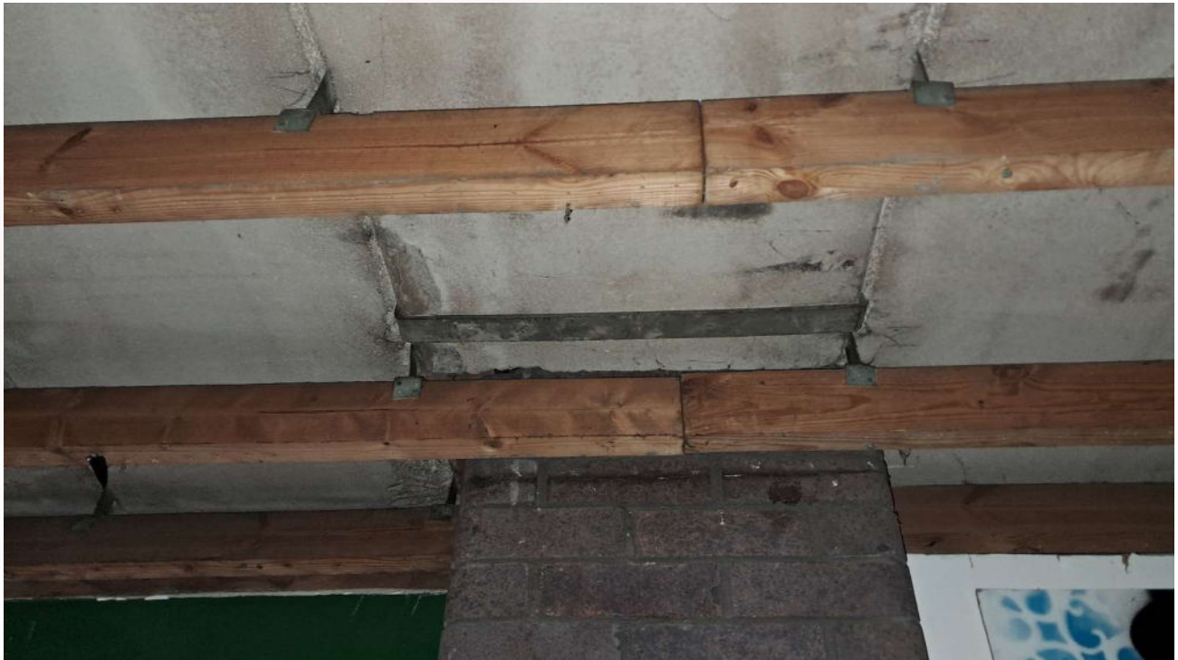
Photograph 45 – typical arrangement of roof abutting column in corridor – staining visible
